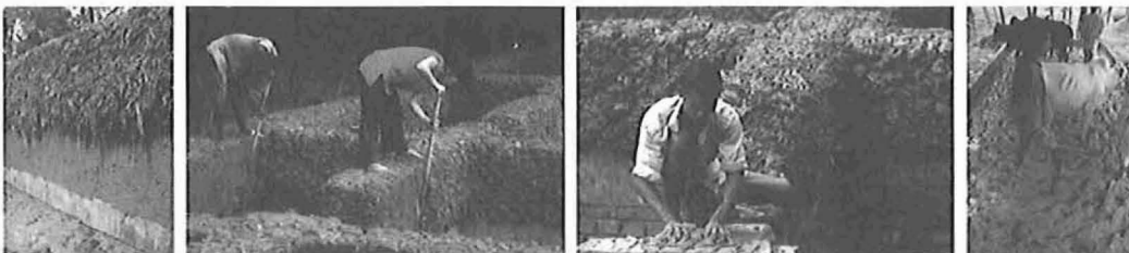
Figure 6 : Source, Anna Herringer, 2007. Weller construction: mixing; placing of first layer, trimming with the spade; 2nd layer (Herringer, 2007)
