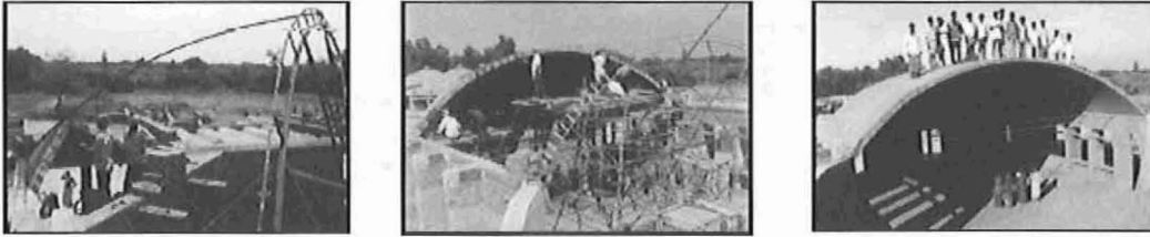
Figure 5 : Segmental vault 10.35m span, 2.20m rise, 6m long, built in 18 days with 4 masons
